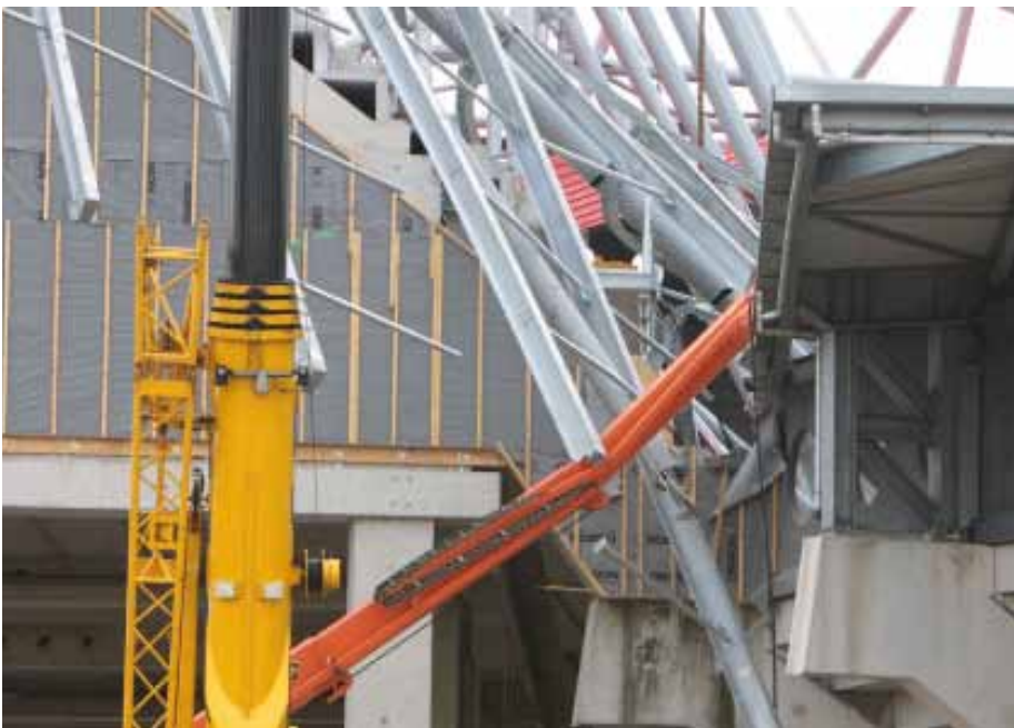
Figure 2 Insufficient stability of roof structure
