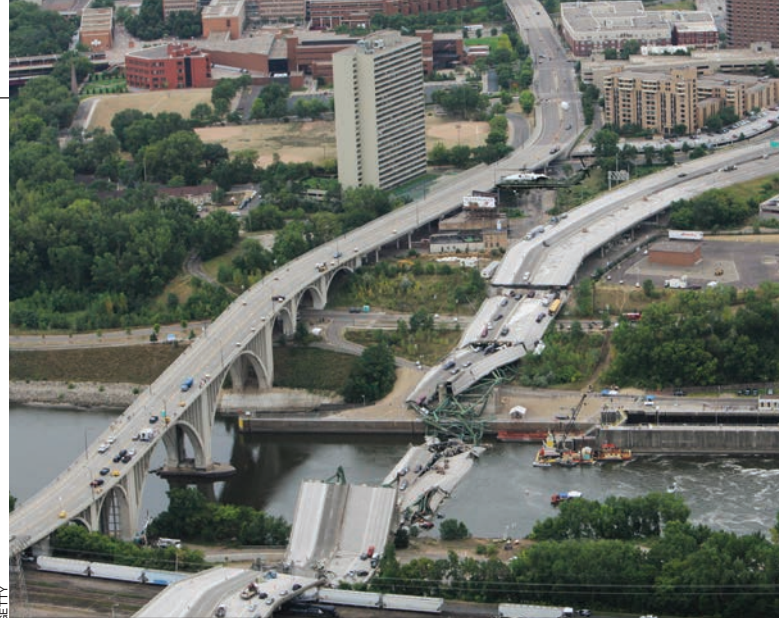
Figure 1 Collapsed section of I-35W Highway Bridge
